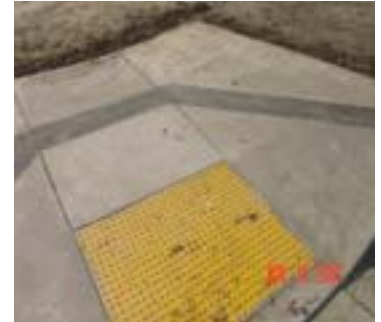
Yellow bumps, called truncated domes installed to assist visually impaired pedestrians.
